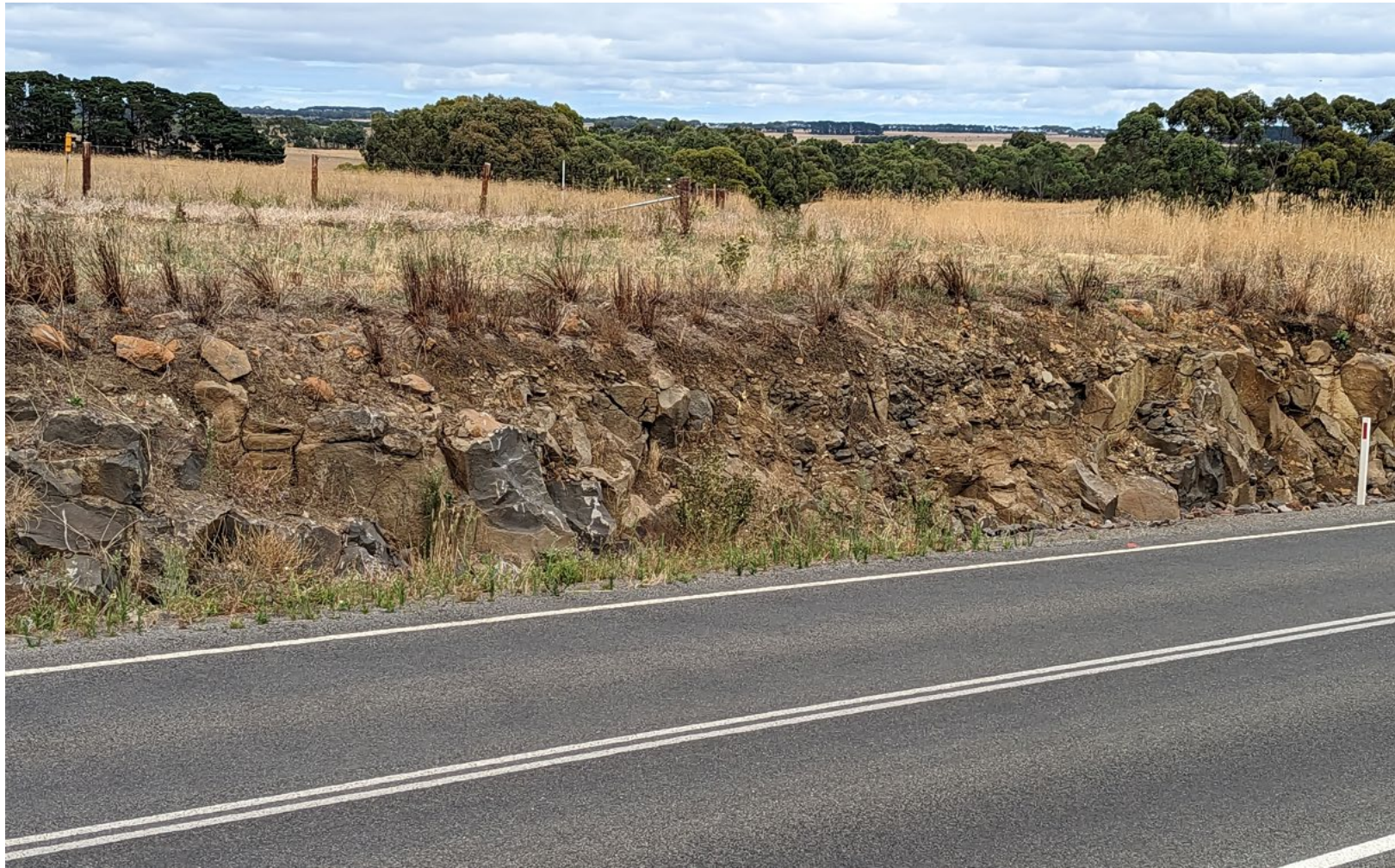
Road cutting on Hamilton Hwy adjacent to Burchett Creek crossing at northwestern site boundary. This shows an example of excavation conditions where basalt rock is close to surface.
