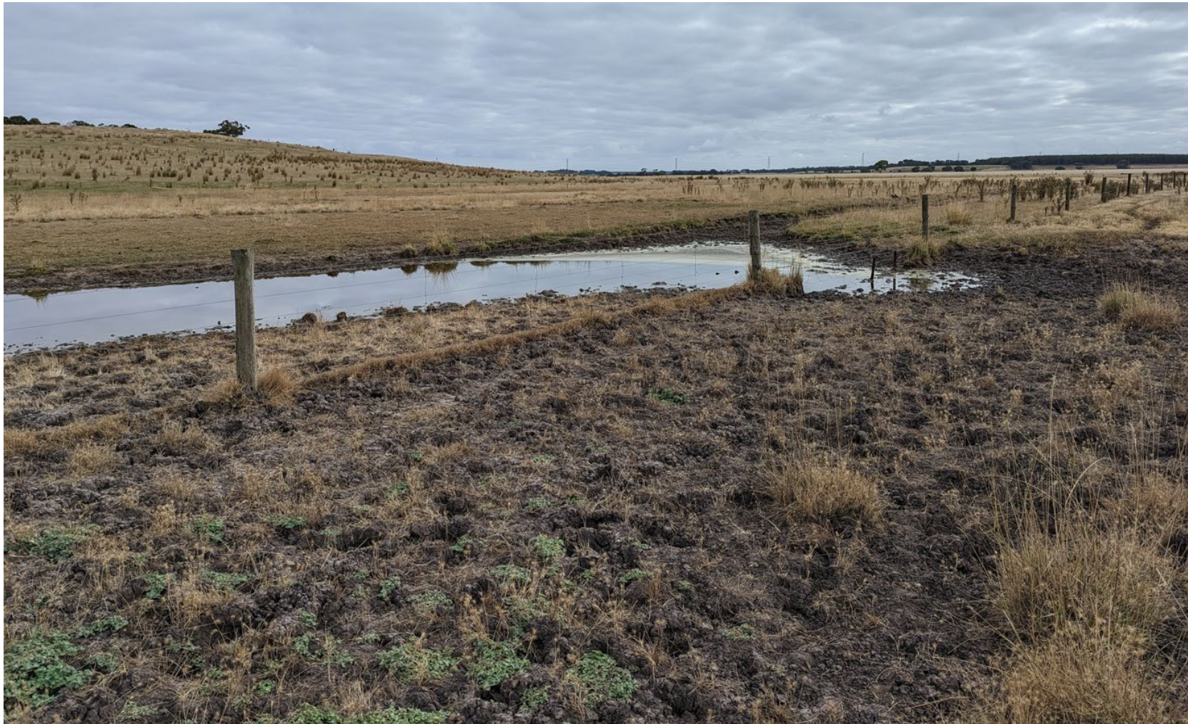
Creek alluvium deposit close to proposed WTG T97. Proposed site access road and underground cable pass through this location. Soil is dark grey, high plasticity clay. Very desiccated. Similar to swamp/lake deposits but may have higher plasticity based on disturbance.
