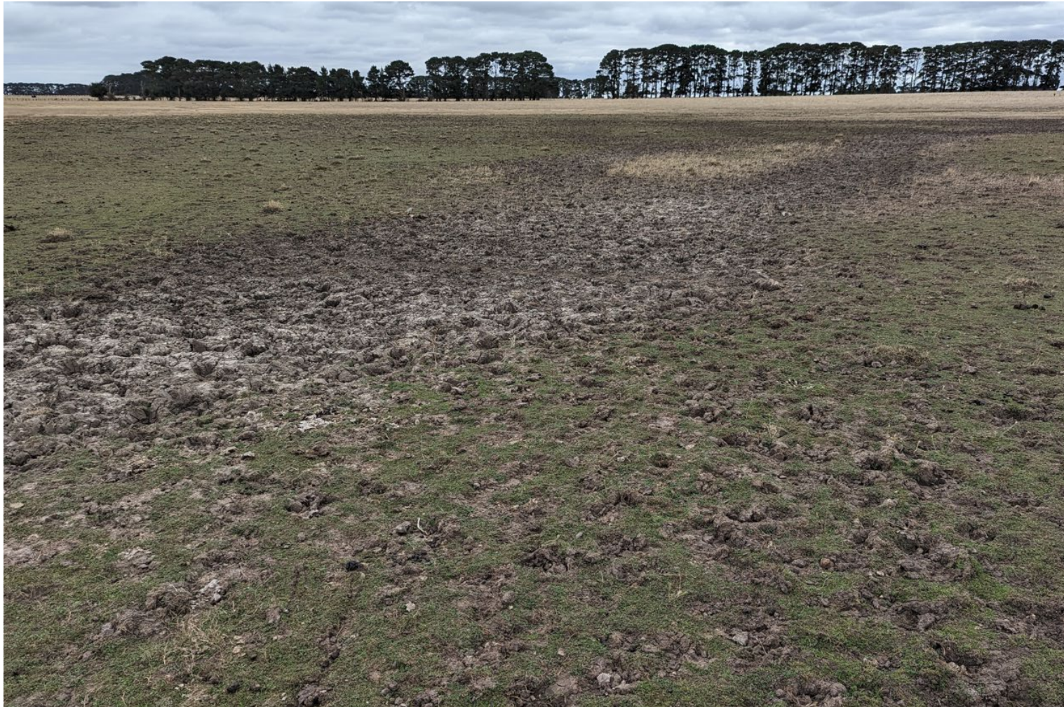
Swamp deposit adjacent to proposed WTG T84. Soil is similar to other swamp deposits but shows a pale grey/white crust at the surface, a potential indicator of salinity.
