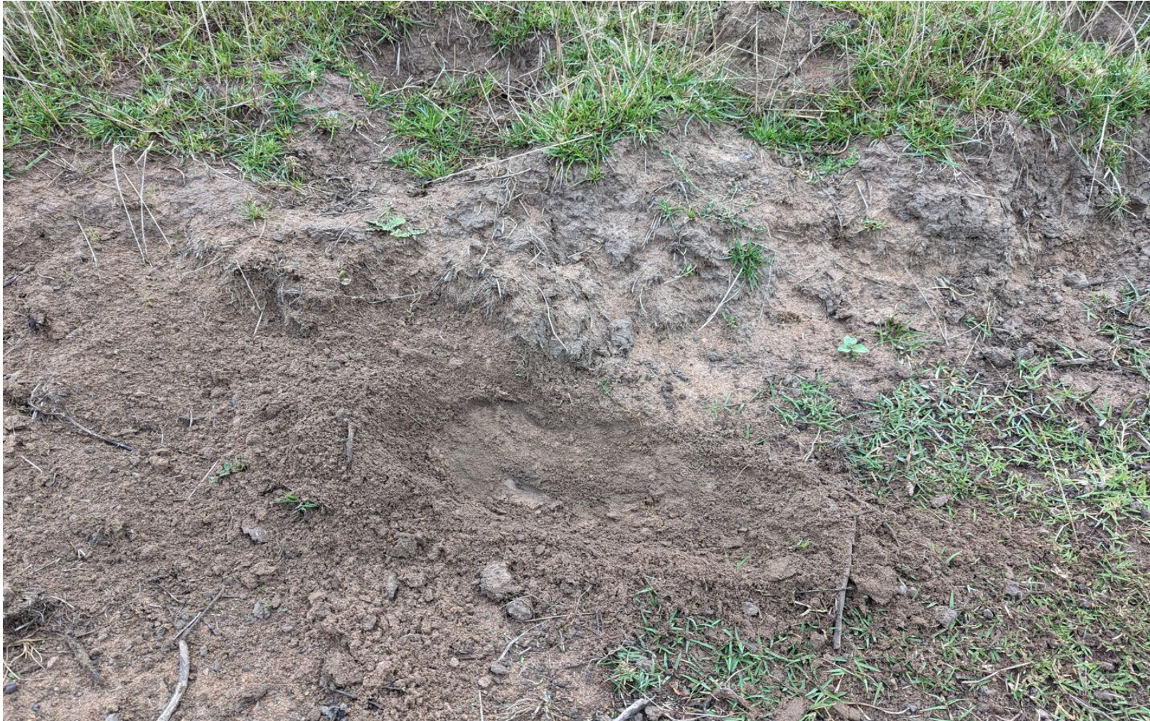
Sandy soil exposed in a swale drain east of proposed WTGs T103 and T105. Consistent with mapped geology showing Brighton Group. Soil is a silty sand with inferred medium dense to dense relative density.
